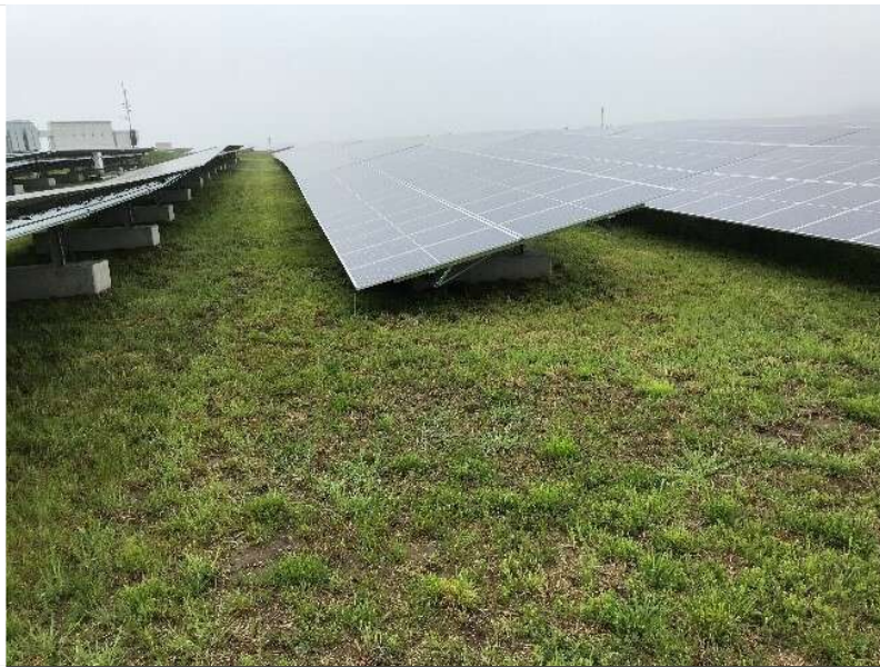
Solar panels at Annapolis Solar Park. The grassy area around the panels could be turned into a pollinator garden.
