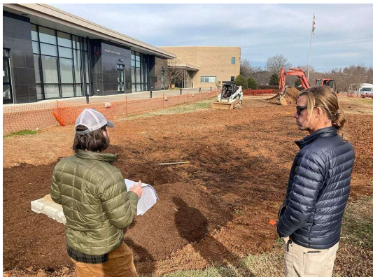
Simon Gregg (left), Kris Bass Engineering Project Engineer, and Robert Osborne (right), Backwater Environmental President, look over the first of two rain gardens during a site visit to the Nash Community College.
