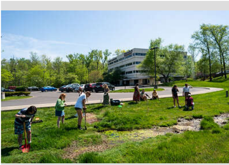
Students working on the installation of a rain garden with native plants on our campus.
